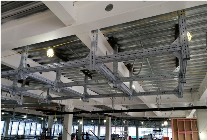
Photo 4; from Wellington Children hospital where frames were restraint design was considered early and suspended frames were used to support and restrain services.
