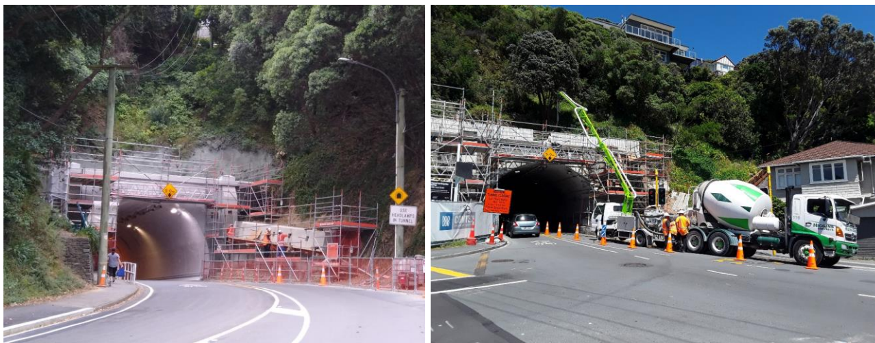
Figure 6: Photographs of the beam construction activities at each end of the tunnel.
