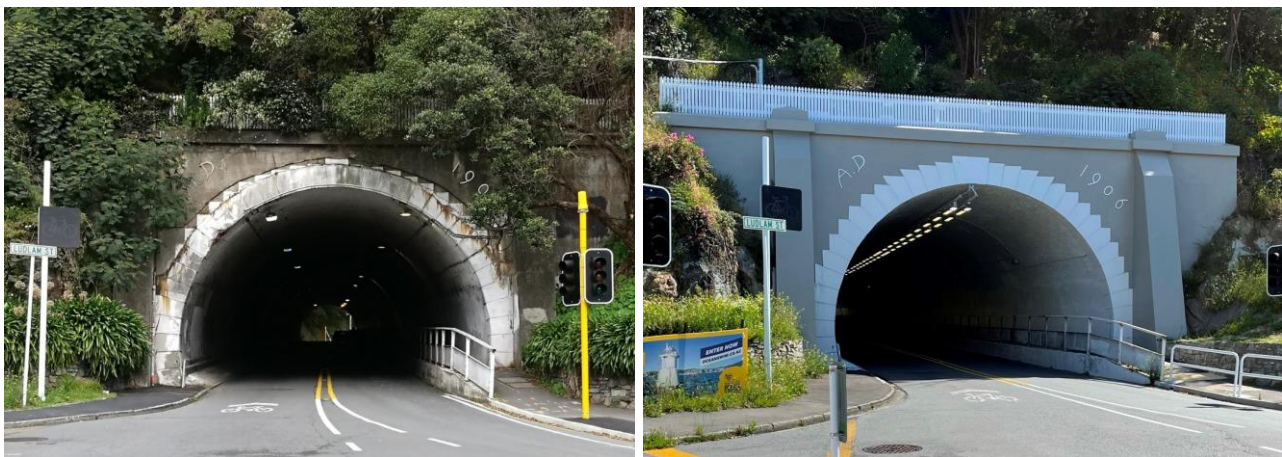
Figure 2: View of the Seatoun portal end, before and after the strengthening works.
