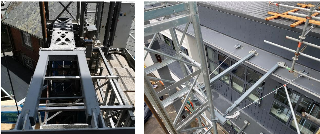
Figure 5: Left - Ductile hoist tie at Bowen House, Wellington. Right – Ductile hoist tie at Wellington East Girls College (courtesy of Naylor Love).
