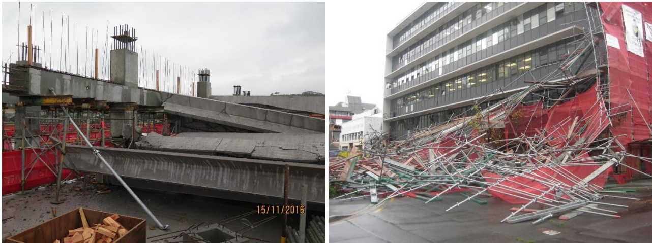
Figure 1: Left: Collapse of precast flooring units on a Wellington construction site during the November 2016 Kaikoura earthquake 2016 (Source confidential, 2016). Right: Collapsed scaffold following the February 2011 Christchurch Earthquake (Coxhead, 2011).
