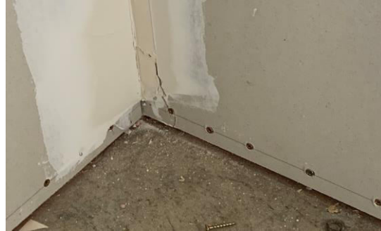
Figure 5. Local plasterboard damage
