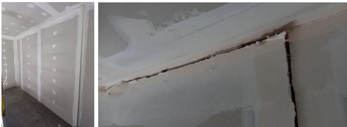
Figure 8. Out-of-plane buckling of plasterboard along the sheet joint
