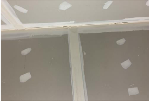
Figure 4. Significant tape breakage
