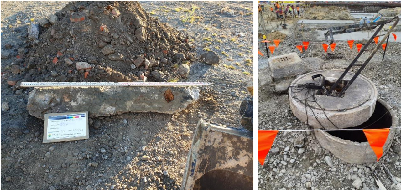
Figure 8. Left - historical foundation beam encountered during enabling works; right - historical oil sump within the foundation footprint encountered during foundation excavation.
