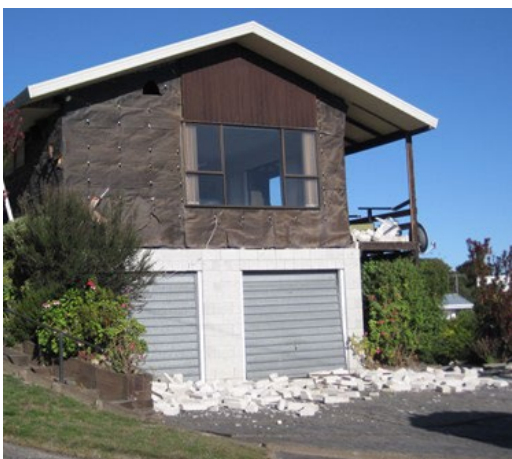
Figure 6: Damage to heavy cladding due to high accelerations during the Christchurch earthquakes (courtesy of Andy Buchanan)
