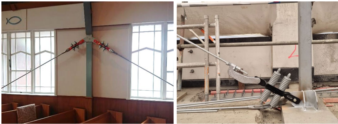
Fig. 4: Samples of the Tectonus tension-only self-centring braces: Tawa Church retrofitting in Wellington (left), and Greys Ave multi-storey bldg extension in Auckland (right)
