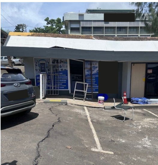
Figure 9. Possible fault rupture through Port Vila CBD. This building was not inspected by the FENZ USAR team.
