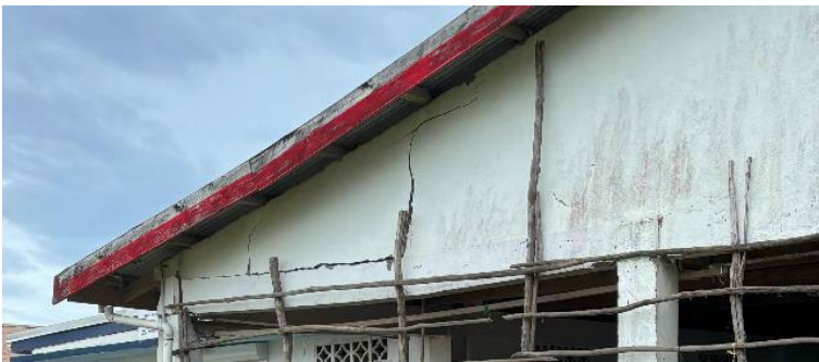
Figure 7. Surface rupture through building. Uplift approximate 300mm. Figure 8. Concrete frame and masonry infill damage as a result of uplift
