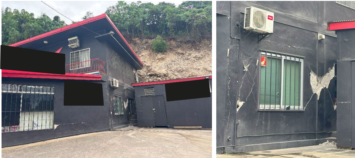
Figure 3 and Figure 4. Landslide behind building. Major damage to concrete columns. Ongoing risk due to further ground movement. Damage to concrete columns and infill masonry due to inertial shaking and impact of landslide.
