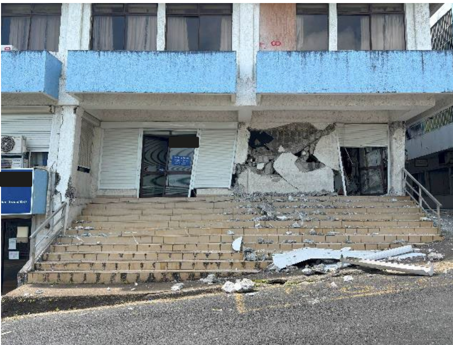
Figure 17. Major damage to ground floor concrete frame and infill masonry wall. Large vertical irregularity with discontinuous frame above entry and potential soft-storey effect.
