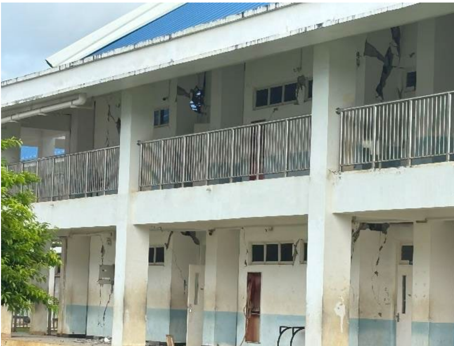
Figure 20. Major damage to infill masonry walls in concrete frame building. No major damage to concrete frame noted, however serious fall hazard from heavily damaged walls and ceilings remains.
