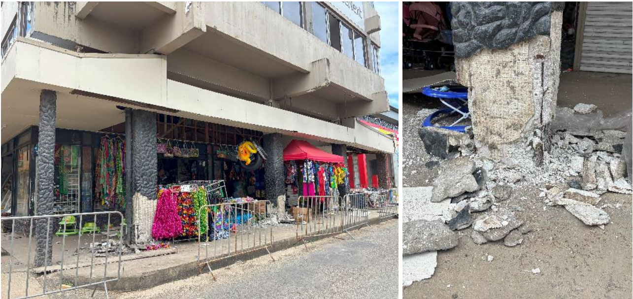
Figure 15. Concrete frame building with major damage to ground floor columns. Likely soft-storey effect due to “tuck-under” parking in the rear and open shopfront in the front.
