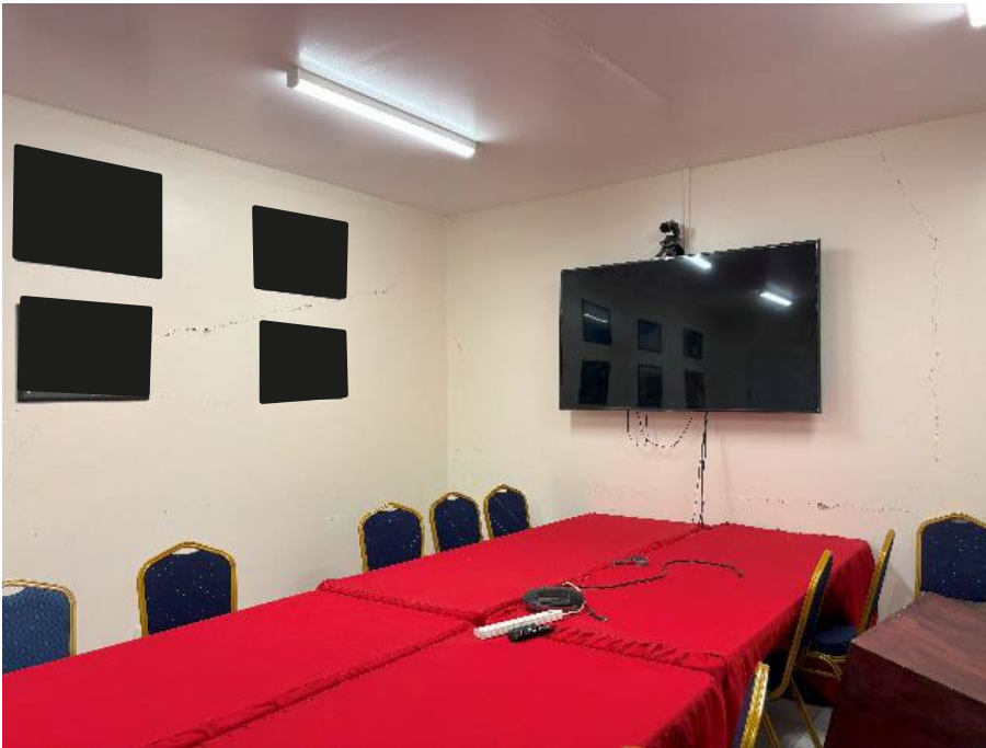
Figure 23. Minor cracks to plaster finish on infill walls. Most common type of damage observed.
