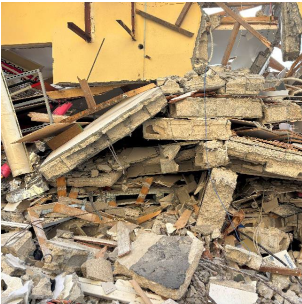
Figure 14. Complete pancake collapse of concrete frame building. Non-ductile concrete frame with masonry infill walls and brittle flooring system with post-tensioned ribs.
