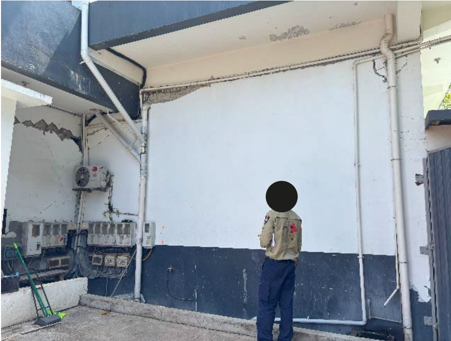
Figure 21. Infill wall damaged at interface with concrete frame. Wall on left verging on major damage due to increasing disconnection from frame and supporting utilities.
