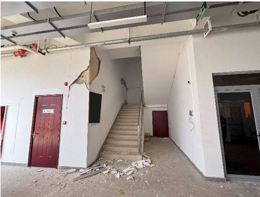
Figure 22. Minor damage to masonry walls at interface with concrete frame. Like many other similar buildings in Port Vila, this building had a thick plaster render applied to the surface of the wall and frame, which failed in a brittle manner before any significant cracking developed in the structure behind.
