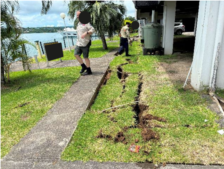
Figure 10. Seawall damage leading to cracking and subsidence next to concrete spread footings.
