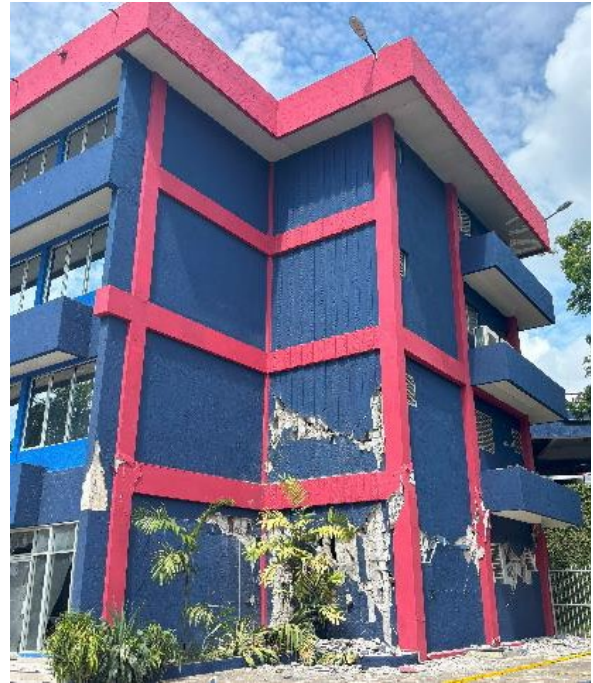
Figure 12. Partial soft-storey collapse of concrete frame building. The building appears to be three seismically separated structures. The left most has suffered a soft-storey collapse at ground level. The other two are also heavily damaged at ground level and above but remain standing with a pronounced lean at ground level.
