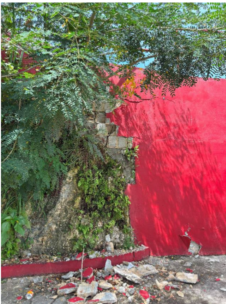
Figure 11. Damage to masonry retaining wall. In addition to the hazard posed by falling blocks, this retaining wall supports a road beyond, which is at risk.
