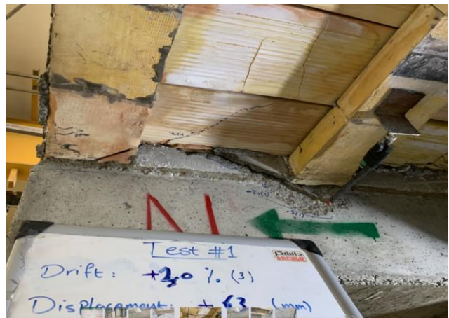
b) Cracking at the Bottom of the Infill Block and the Corner of the Rib Plank
