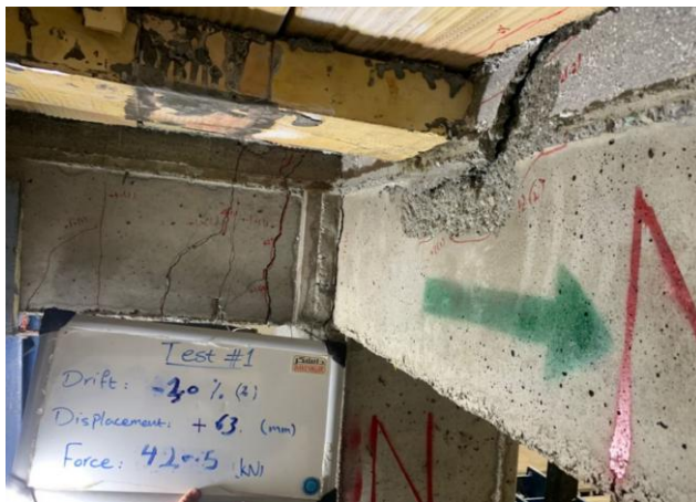
a) Rib Pull-Out Observed at 3% Drift
