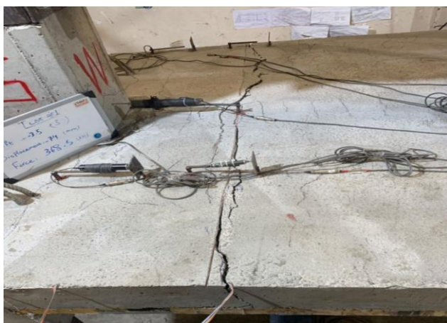
c) Mesh Failure at 3.5% Drift (West Side)
