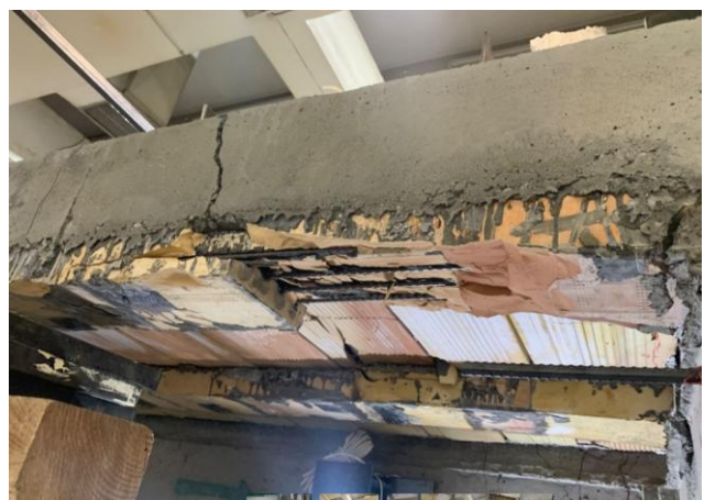
d) Rib Negative Moment Failure and Prestressed Plank Separation at 3.5% Drift (West side)
