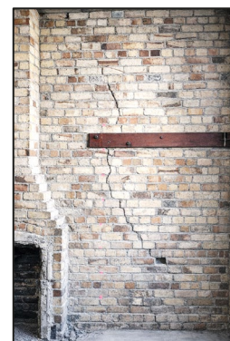
(b) Differential settlement cracking
