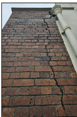
(a) Thermal expansion cracking
