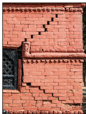
(b) Earthquake cracking
