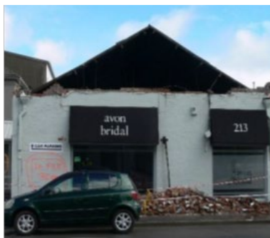
(a) Concrete lintel discontinuity
