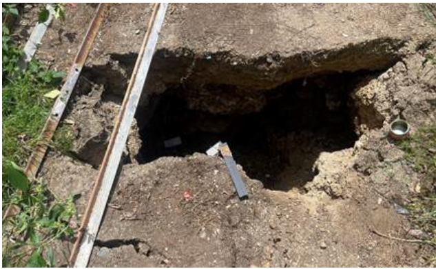
Figure 4: Wharf road landslide behind crest slope failure
